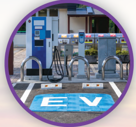
EV Charging Station
